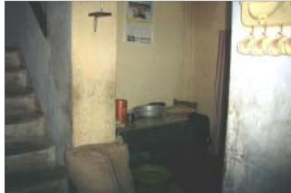
Figure 5.49: The new dining place. This new addition blocking the natural light and ventilation.
